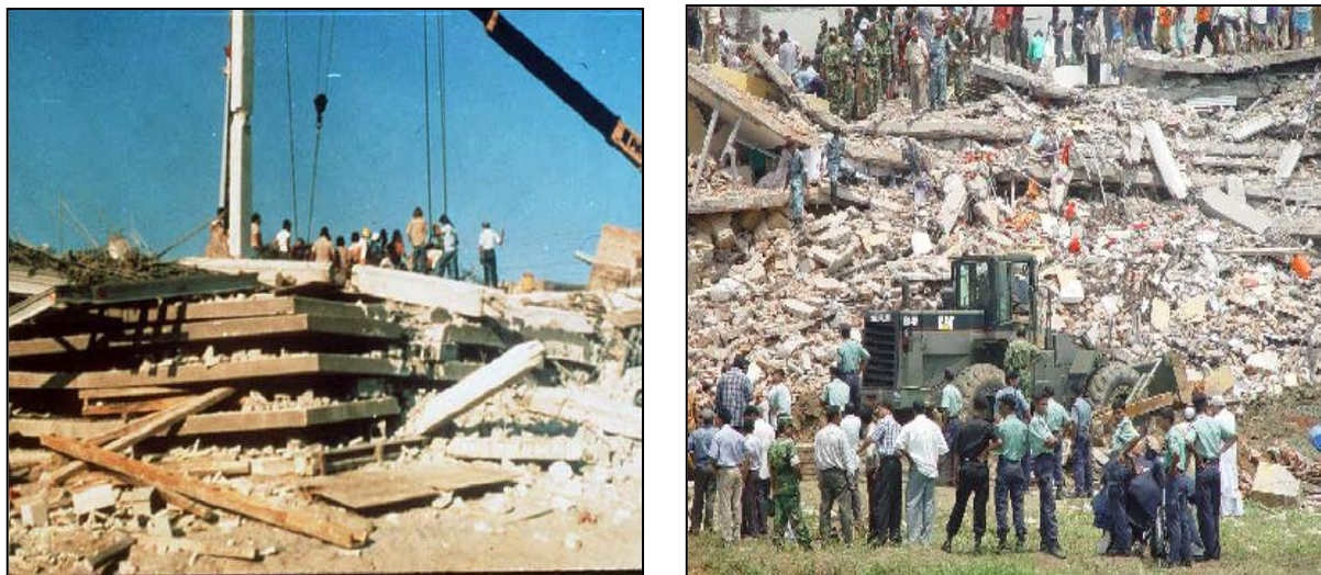
Fig. 8: Progressive Failure of slabs in (a) USA (1981), (b) Bangladesh (2007)
