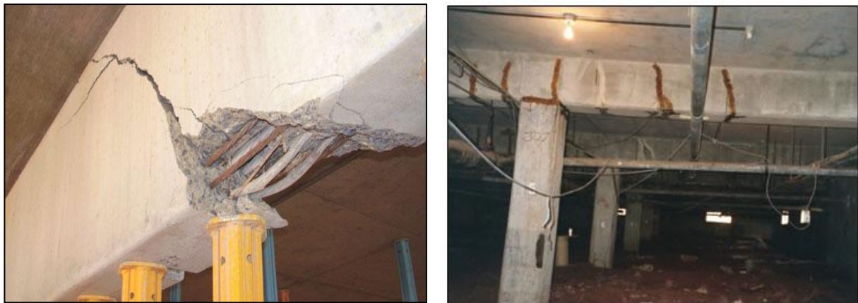
Fig. 2: Various cracks developed in beams and columns due to overload
