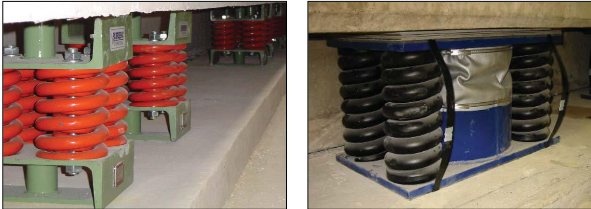
Fig. 19: Machines supported on shock-absorbing springs
