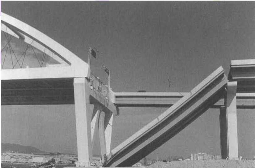
Unseating of simply supported link span in the 1995 Kobe earthquake
