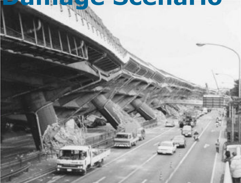
Flexural failure at the base of bridge pier of the Hanshin expressway in the 1995 Kobe earthquake
