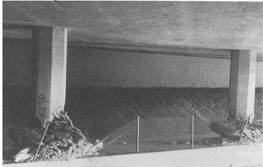
Failure of flexural plastic hinges in bridge piers in the 1994 Northridge earthquake
