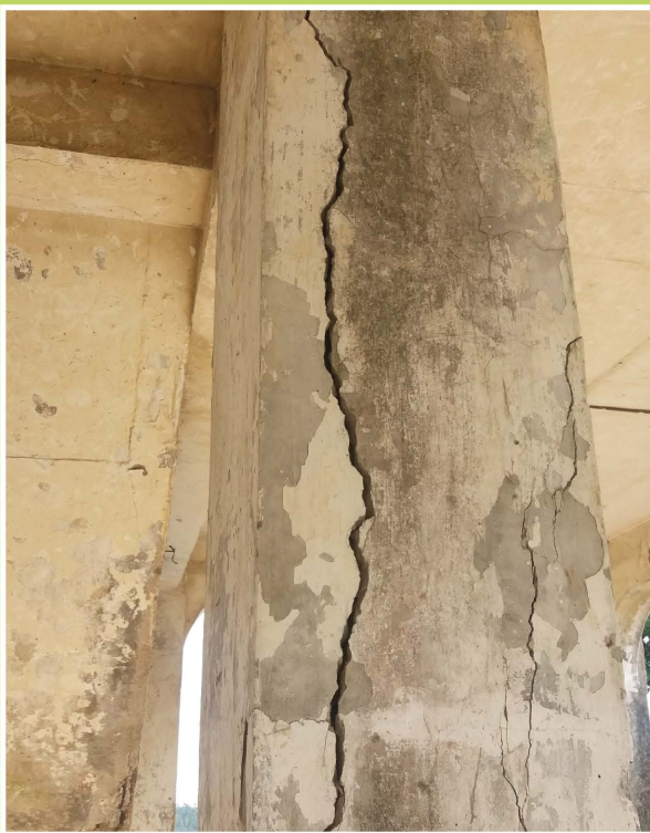
Spalling of concrete cover due to de-bonding induced by rebar rusting
