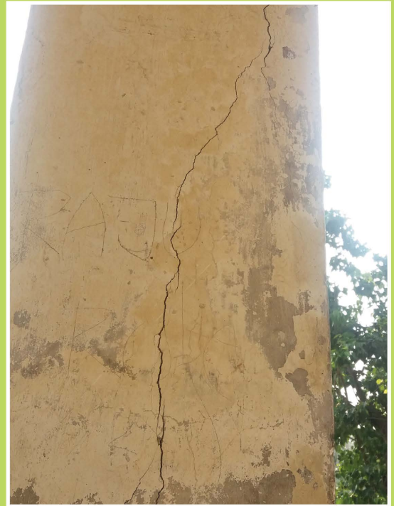
Cracked concrete column due to rebar rusting
