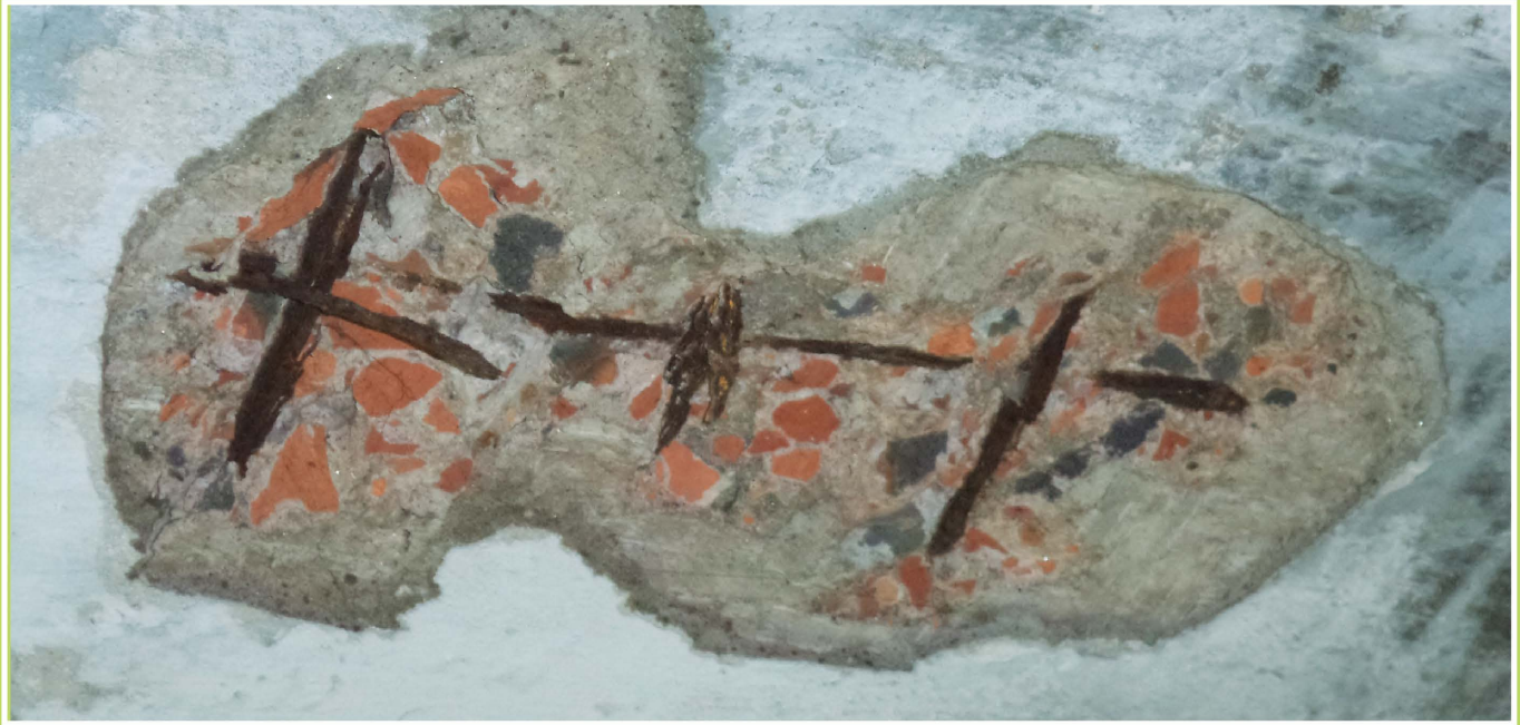
Cracked Concrete Ceiling
